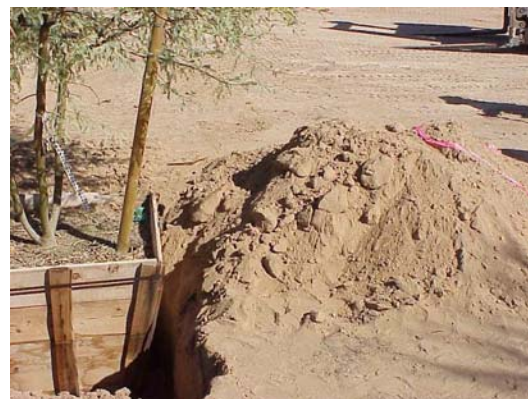
Figure 6. Back fill with the soil removed from the hole to create a good interface between the rootball and the surrounding undisturbed soil.
